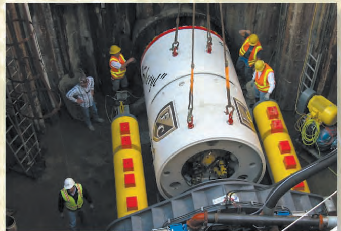
Bohrkopf in Pressstation, Seattle, USA / Cutter head in jacking rig, Seattle, USA
